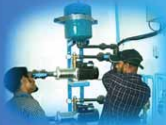
Trading activities - Booster pump system to provide high pressure water above 4th floor in high rise buildings
